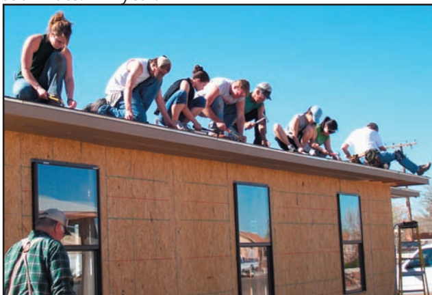
North Dakota State University students "hammer down" on the roof at 1436 N. Second St.
